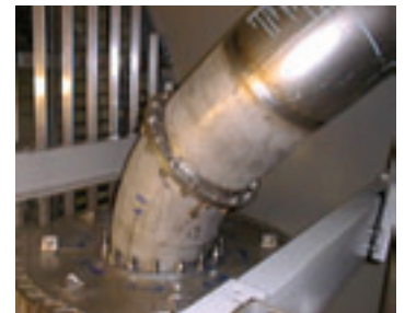
Top View of Installed ZSQ Inlet Device
